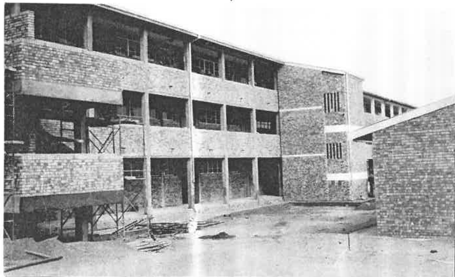
Above: Building of the new Umso Secondary School. The building is still under construction, but is expected to be completed by the end of next year.
