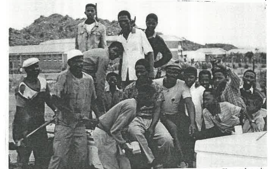
Here members of the Civics Association are at work building humps in Kuyasa's main street to curb fast driving and protect pedestrians.
